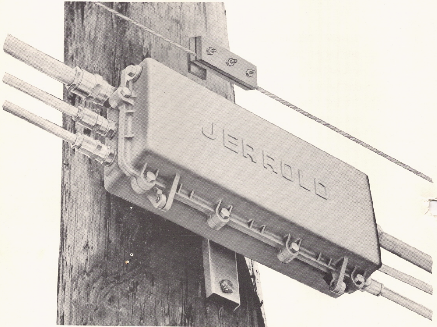
Fig. 1. Main Trunk Station, Pole-Mounted
